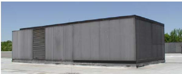
Enclosed Rooftop Chiller System
